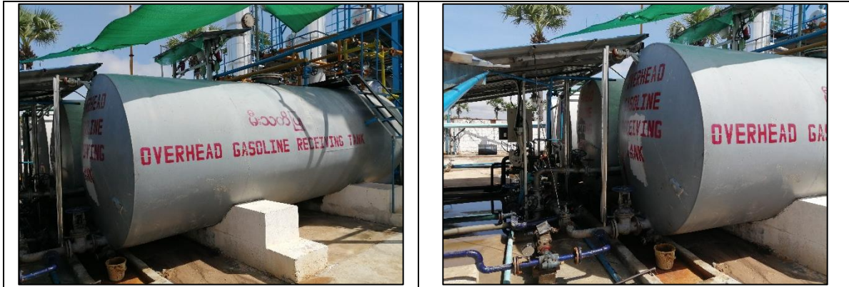
Figure 3-11 Overhead Receiving Tank
