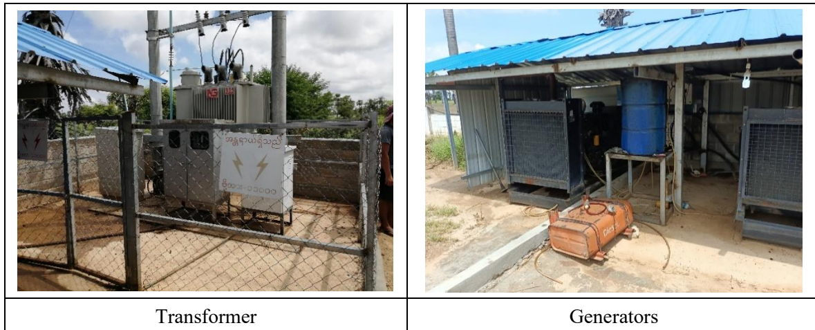
Figure 3-18 Electric Supply System (Transformer, Generator)
