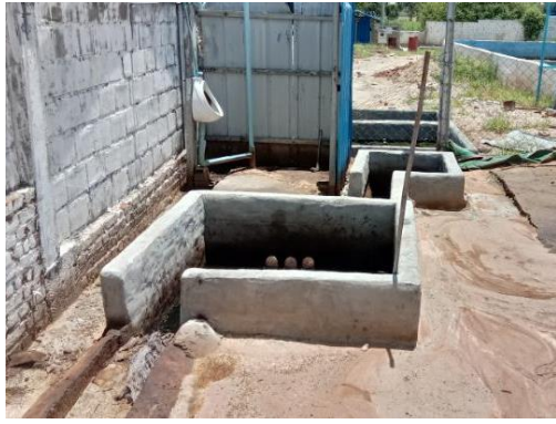
No 1 and 2 (Oil filtration tanks)
