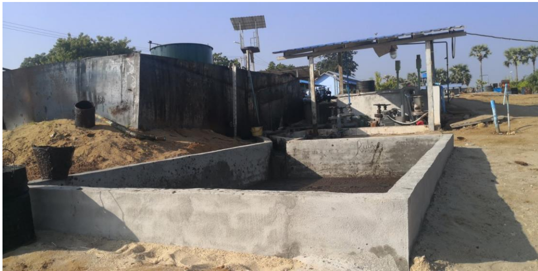
No.4 (Water treatment tank)
