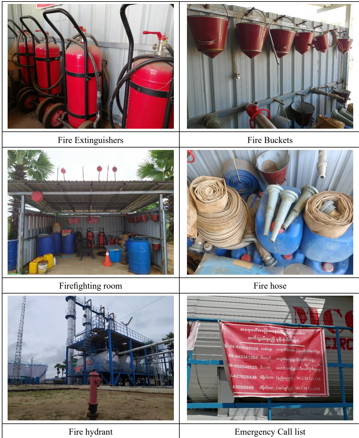
Figure 3-35 Fire Safety Facilities
