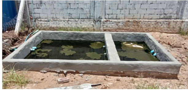
No.3 (Water filtration tank)
