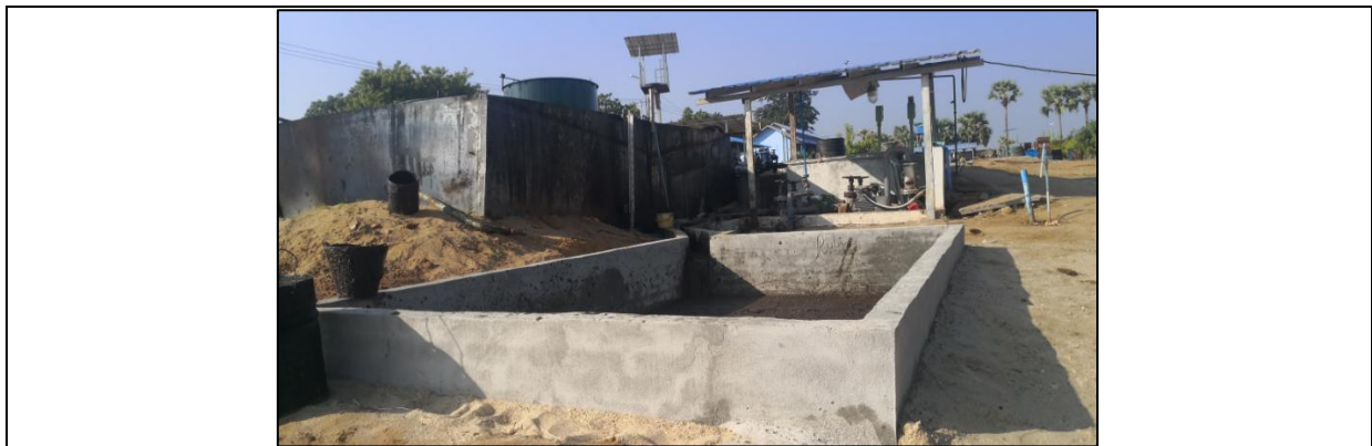
Figure 3-6 Water stored tank
