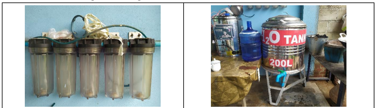
Figure 3-32 Photos of Drinking Water Facilities
