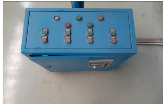
Assembling Line Control Unit
