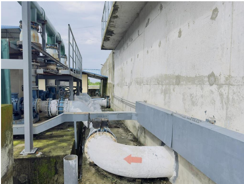
Photo 3-12: Exit pipe from sedimentation tank
