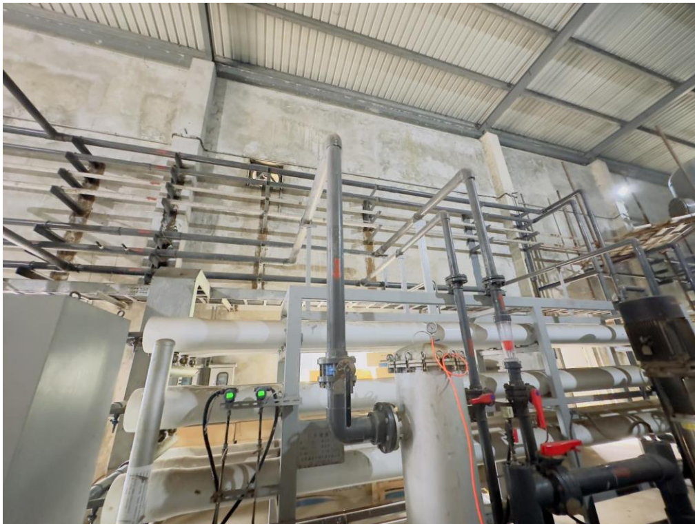
Photo 3-20: Reverse Osmosis System (1)
