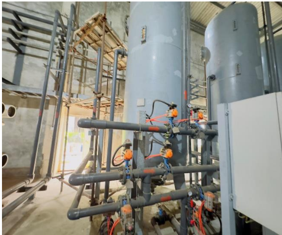
Photo 3-23: Entering pipe to cation column
