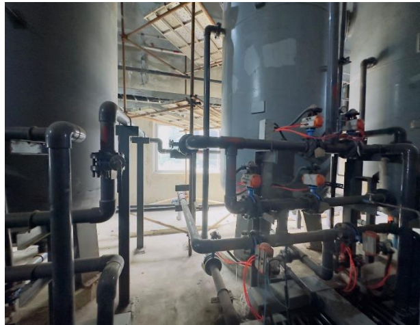
Photo 3-24: Exit pipe from cation column and enter pipe to anion column
