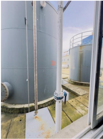
Photo 3-18: Enter and exit pipelines at ultrafiltration tank
