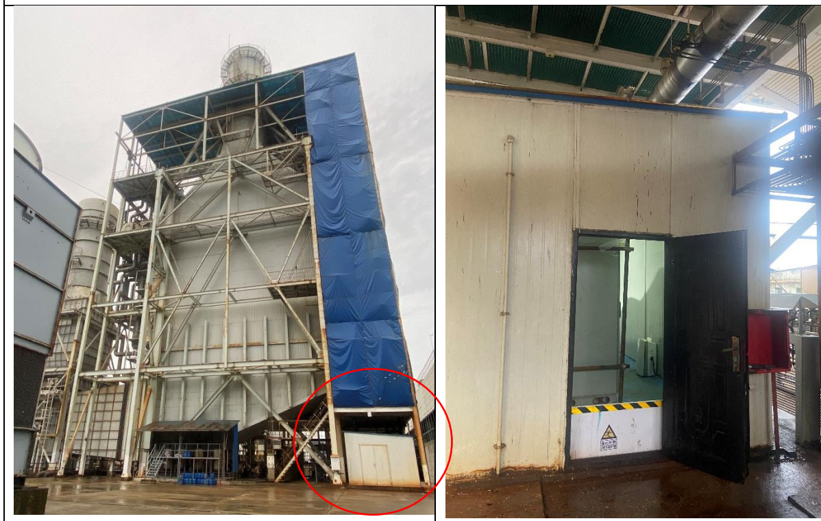
Gas Analyzer Control Room
