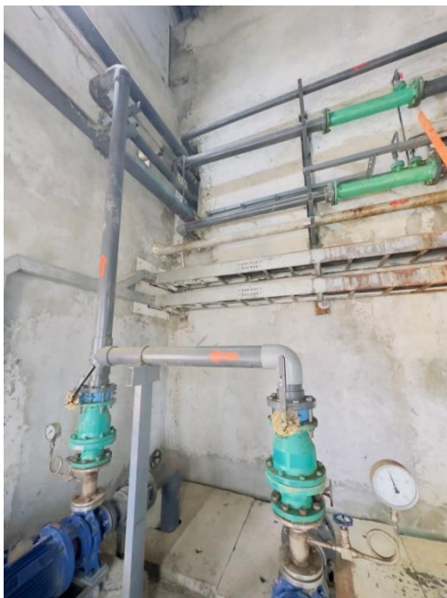
Photo 3-16: Exit pipes from raw tank connected with pumps
