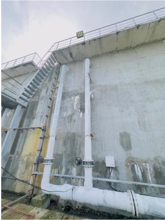
Photo 3-10: Sedimentation tank and water enter line
