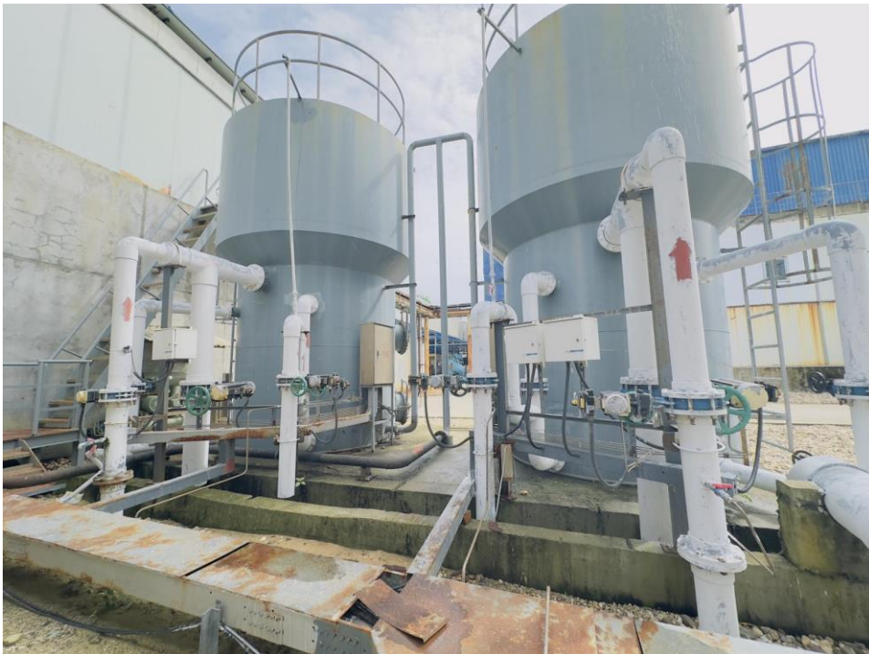
Photo 3-14: Sand filters and exit pipes
