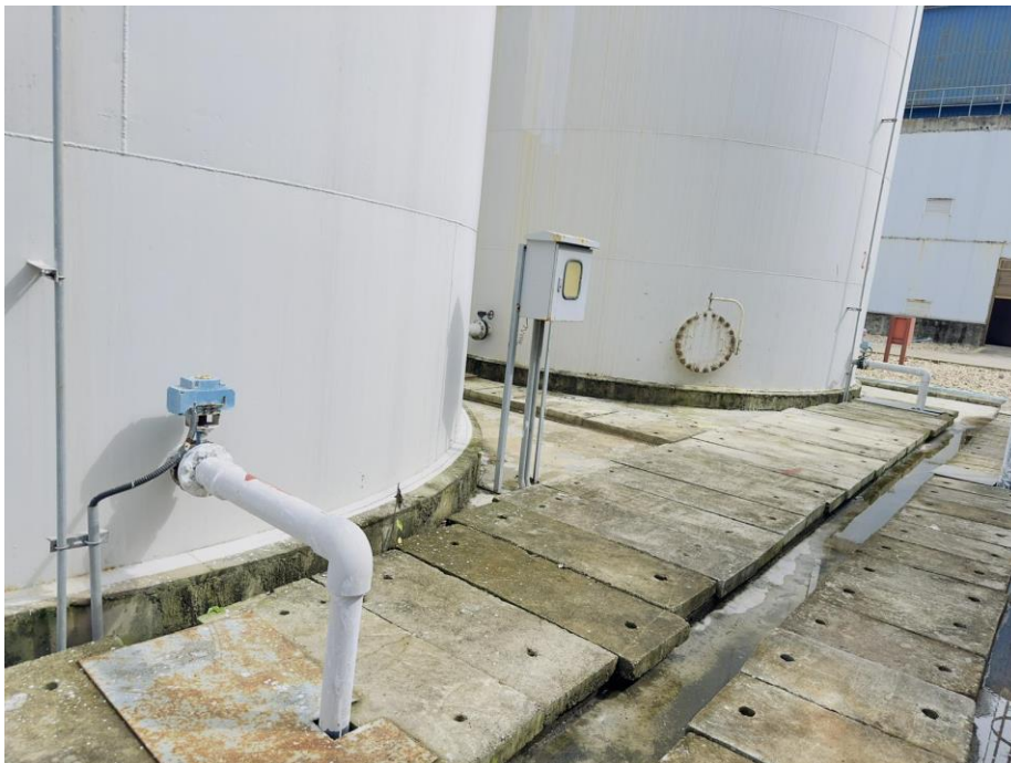
Photo 3-22: Pipe lines enter demineralization tank
