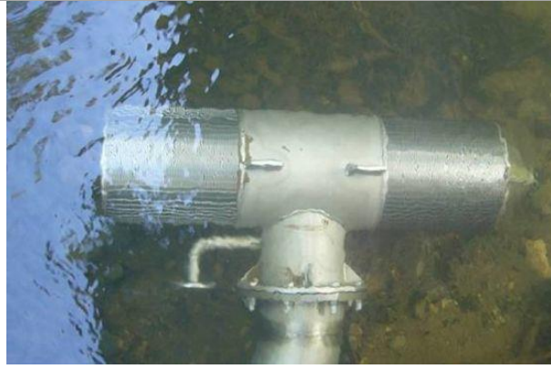
Photo 3-3: Water Intake Screen 6
