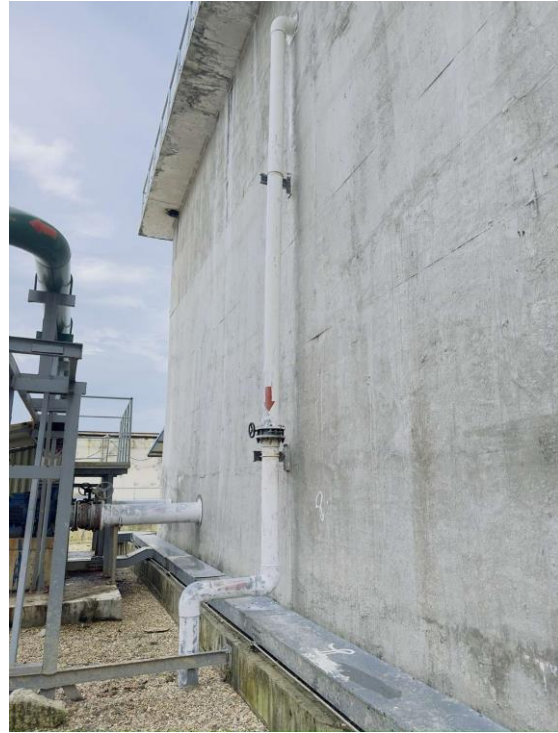
Photo 3-11: Sedimentation tank and exit pipe
