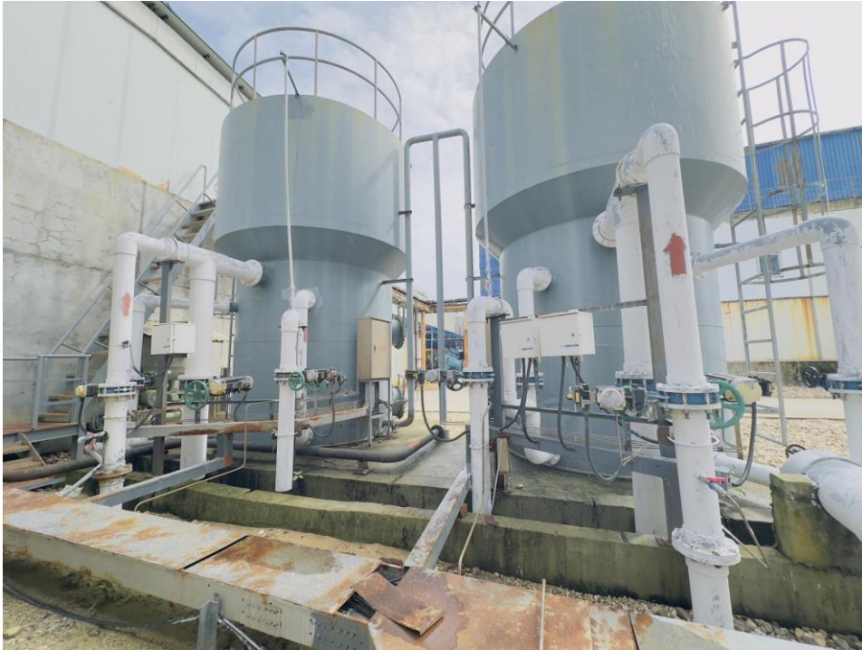
Photo 3-13: Sand filters and enter pipes
