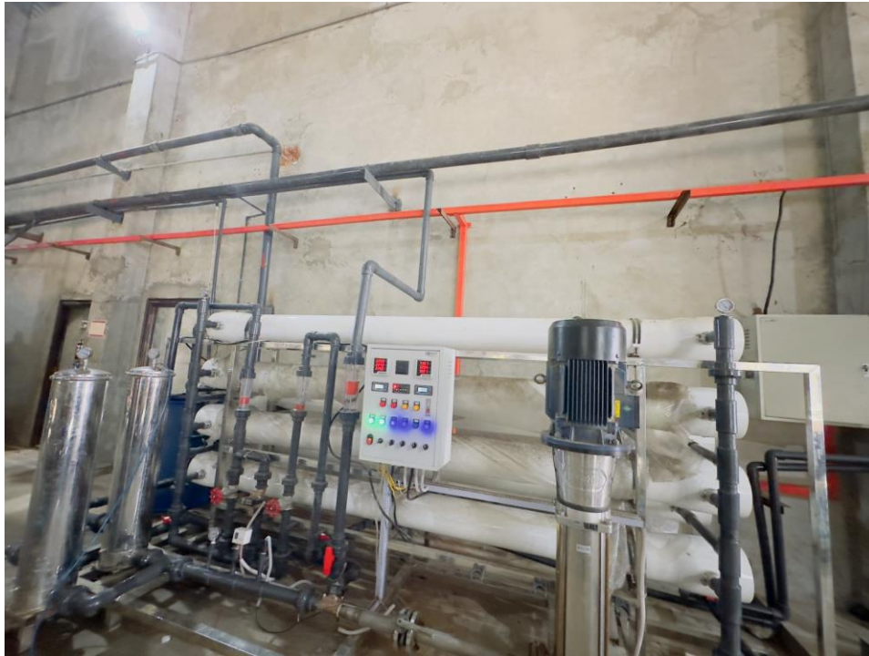
Photo 3-21: Reverse Osmosis System (2)
